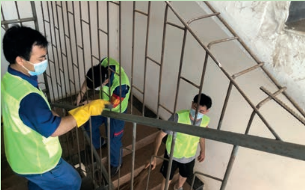
Volunteers helped to renovate the stair handrails, gates and other public facilities of the village committee office building in Nabo Village
