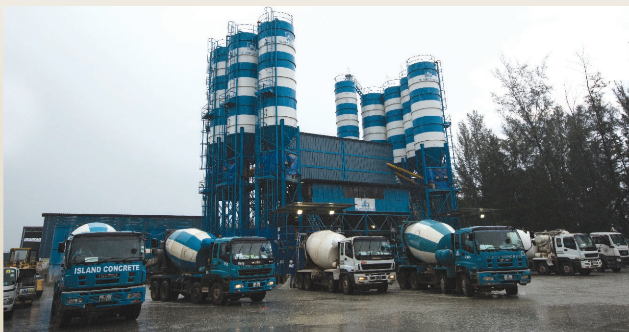
A concrete batching facility of Island Concrete Pte Ltd.
